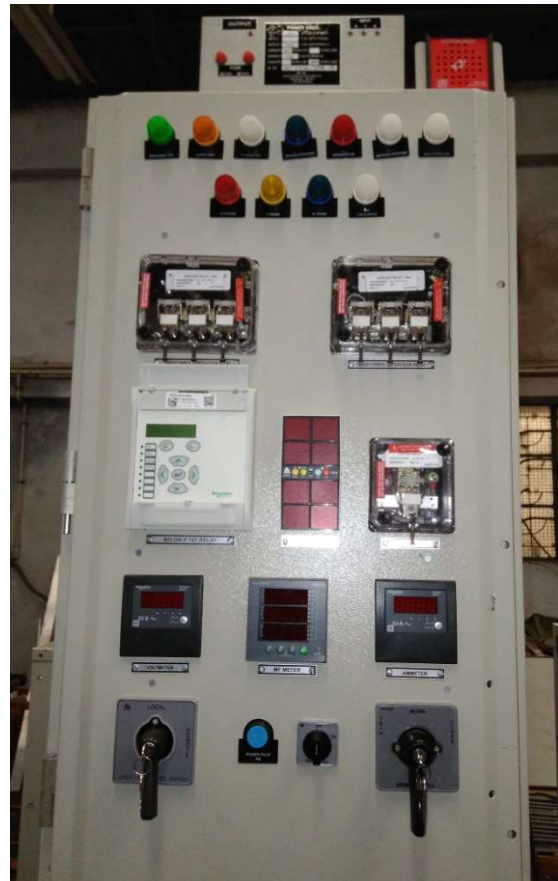
11KV Instrument Chamber
