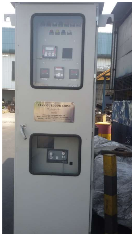
11KV Outdoor Panel
