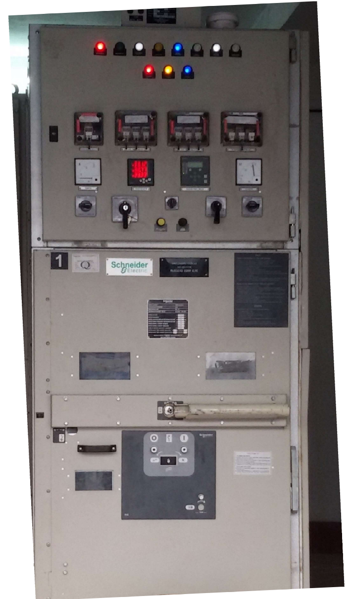
33KV Indoor Panel
