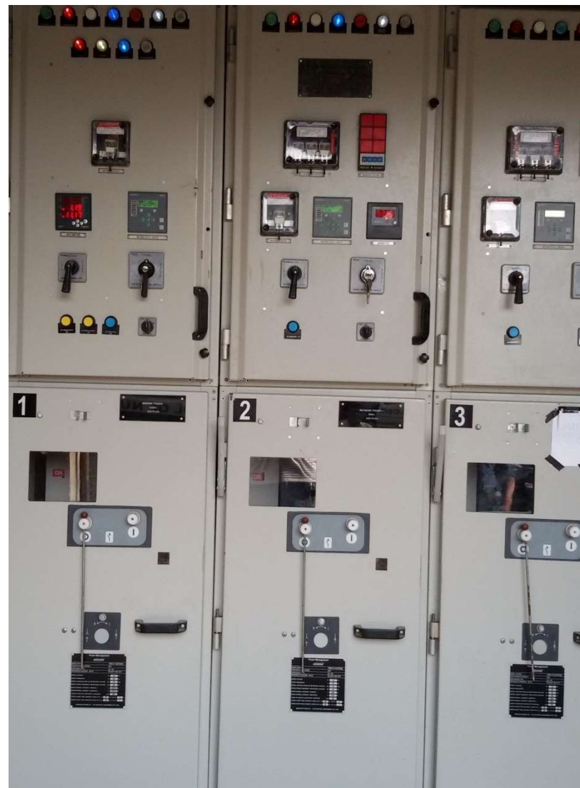
11KV Switch Board
