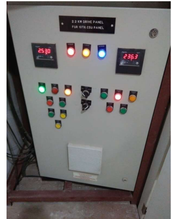
2.2KW Drive Panel
