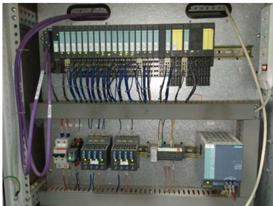
PLC panel internal wiring
