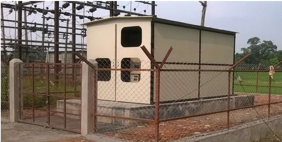
33KV Outdoor Panel
