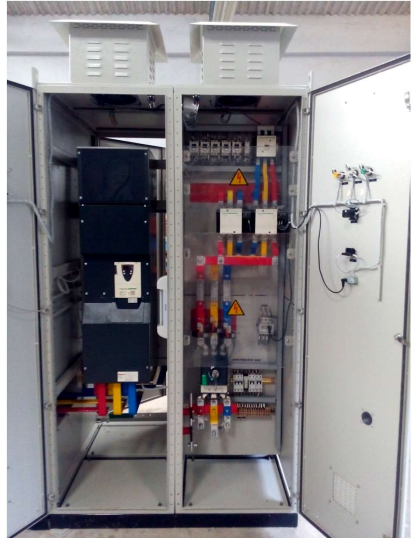
160KW Drive panel
